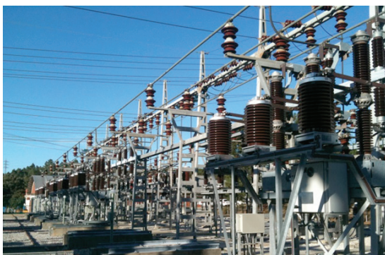
WSAN4CIP demonstrator in a substation of the electricity distributor EDP in Portugal
